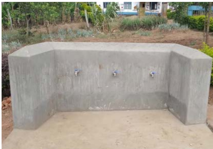
A fill station with spigots on the wall
