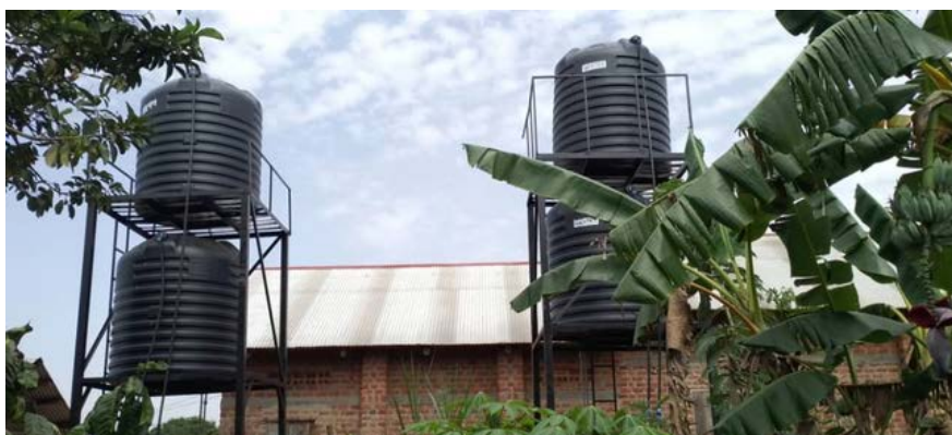
Water storage tanks to hold clean water for the community
